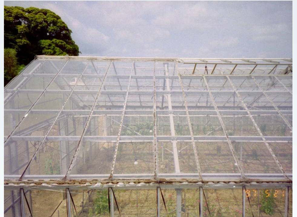
Greenhouse in Kyushu installed in 1988, photographed in 2008.
